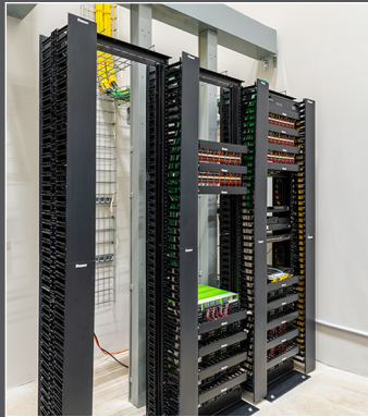
Headends include servers, network switches, and transmitters connected with Remeë's PowerPipe™ Class 4 FMP hybrid cable to provide power, connectivity, and control for the PoE lighting system at Mouser Electronics.
