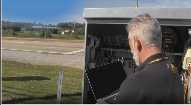
Activate™ by Remeefiber optic cable interconnected the processor with the bell camera.
